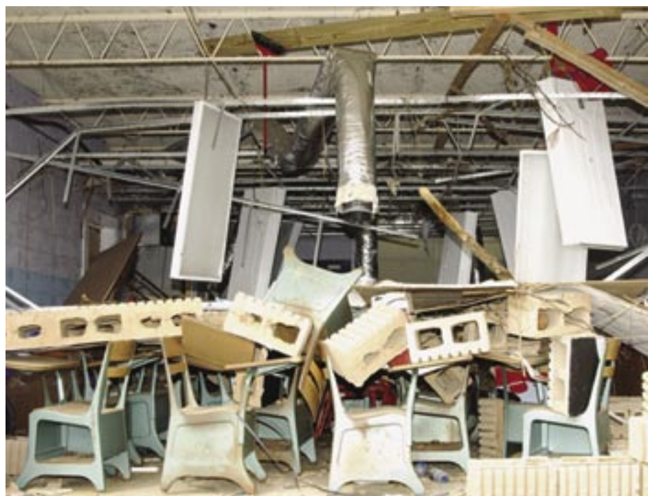
Damaged school in Jackson County School District, Mississippi
